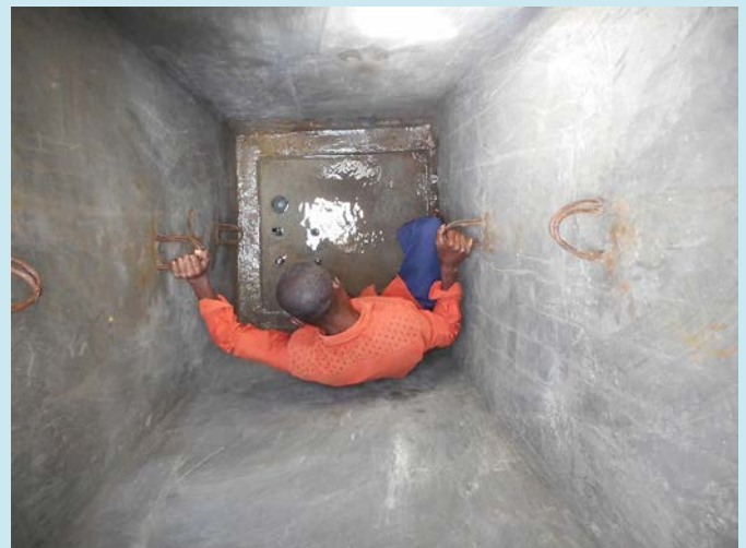
Spring Catchment Box Inside View
